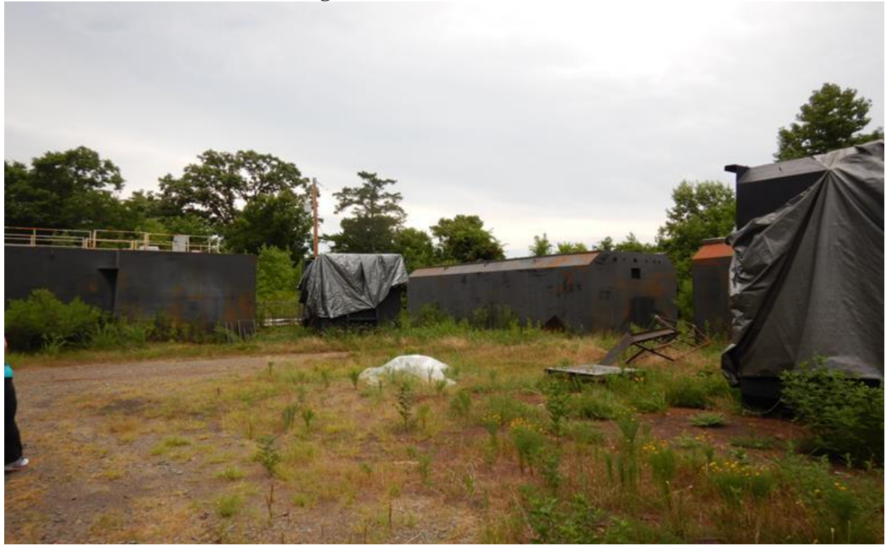
Package Wastewater Treatment Plant
