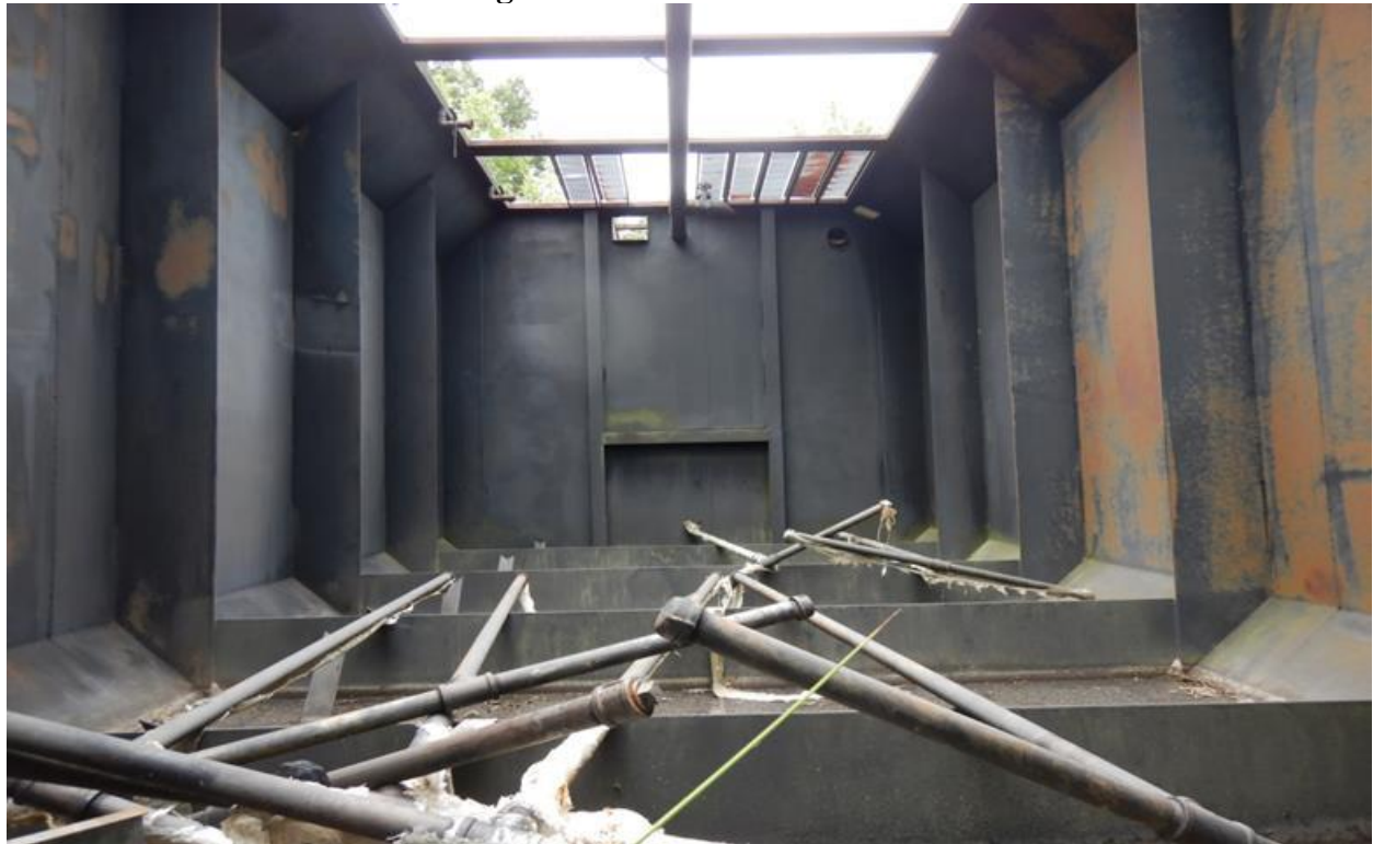
Package Wastewater Treatment Plant
